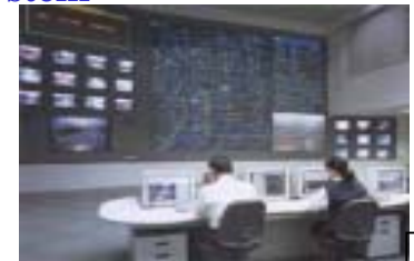
Traffic/Road Management System
