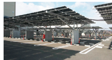
Carport type solar power generation system
